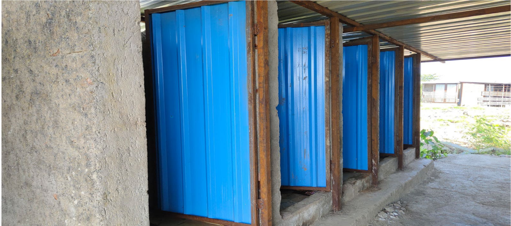
Labour Camp Toilet Arrangements
