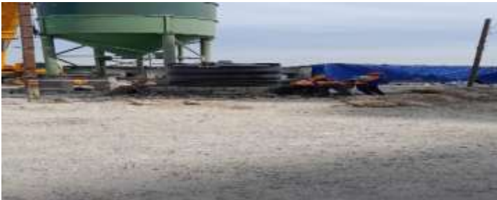
construction labour - drinking water facilities provided.- (R.O. Plant)
